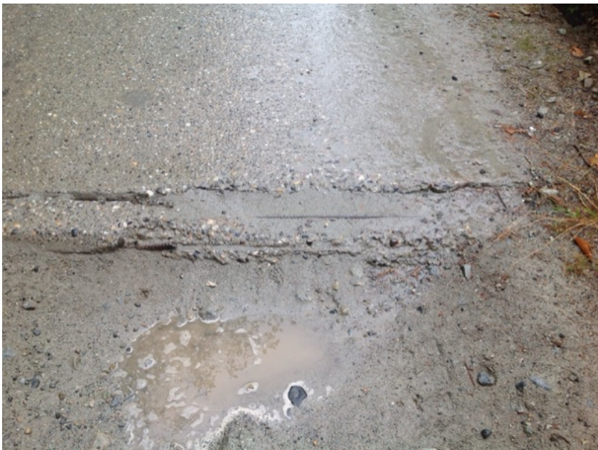
right bank ballast all damage
